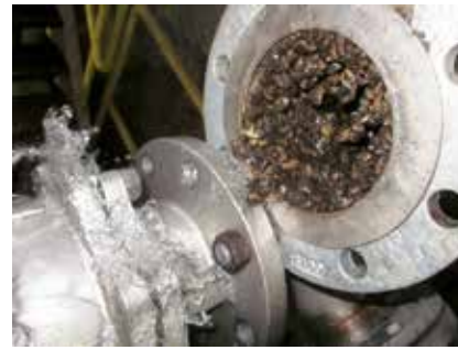
Zebra Mussel Colony in a Pipe. Photo courtesy of Chapman Marine Inc.
