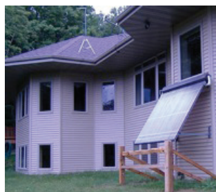
Evacuated Heat Pipe Solar Collector
