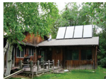
Flat plate collectors for SHW and Space Heating
